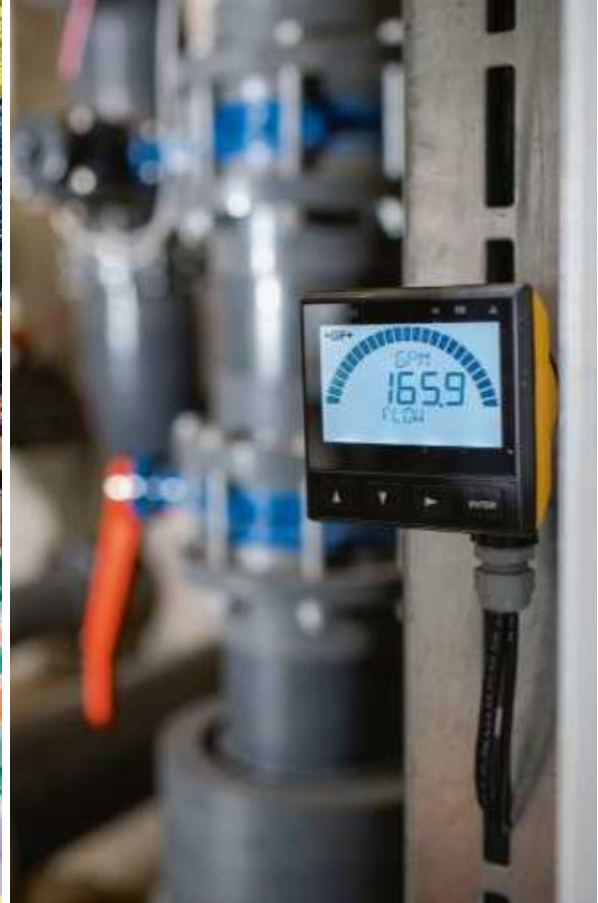
With GF Signets 9900 Transmitter, all relevant water parameters are visible at a glance.
