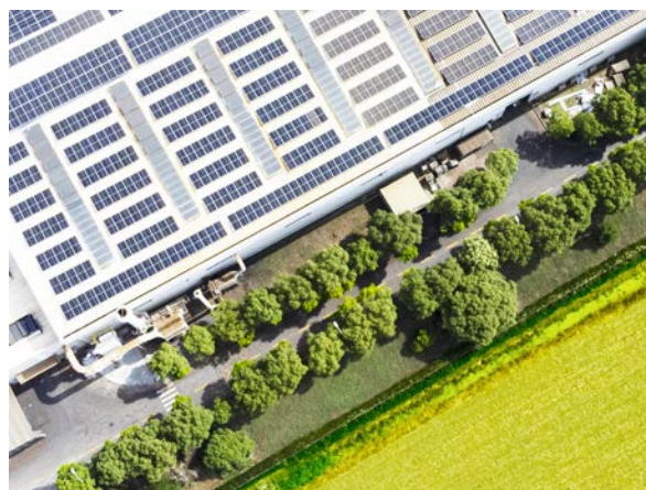
GF Casting Solutions installed 2.0 MW of roof-mounted PV capacity, such as this 1.4 MW system on the iron foundry in Kunshan (China).
